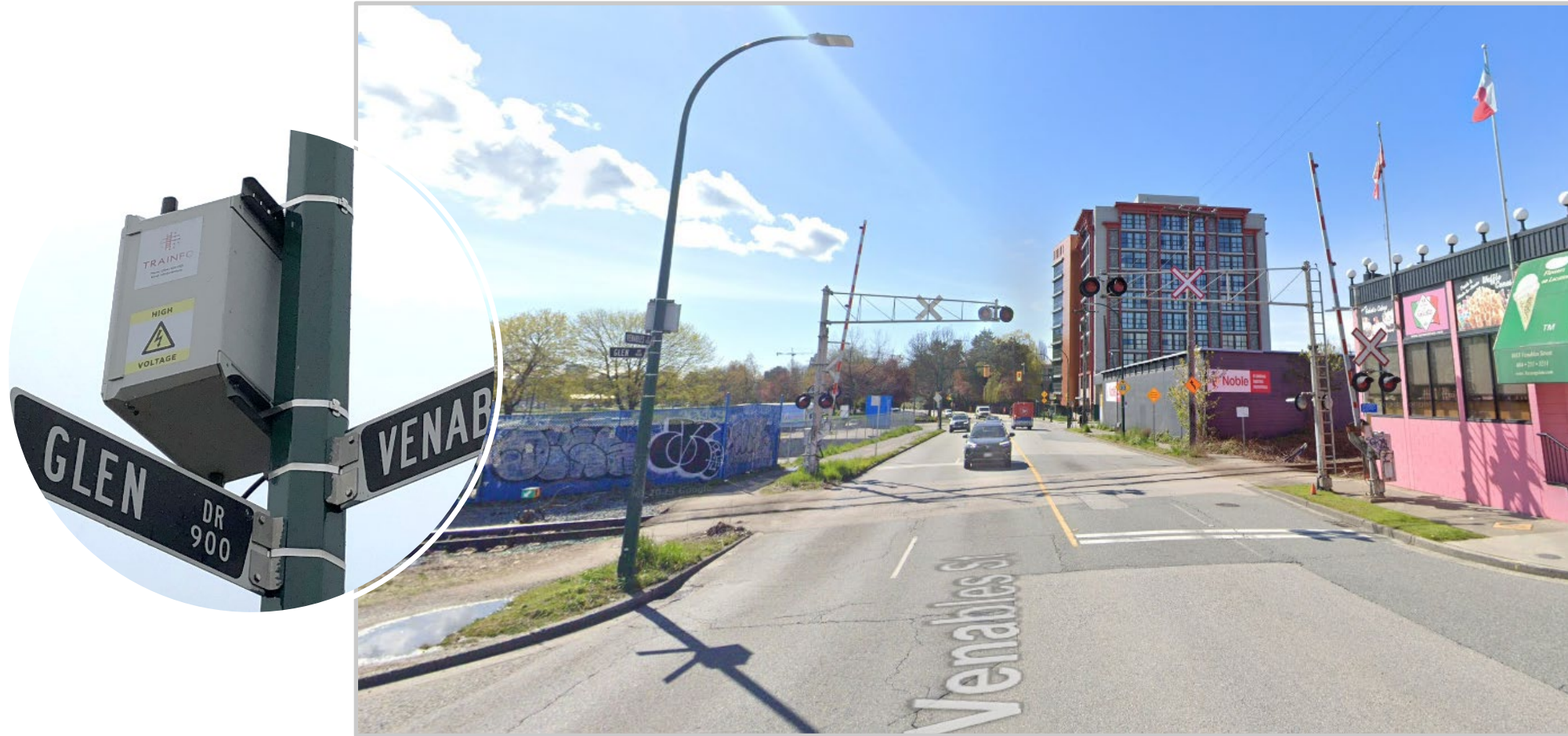
Train sensor at Venables St rail crossing
